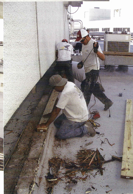
An Insulated Roofing Contractors crew replaces the roof system's existing expansion joints.
